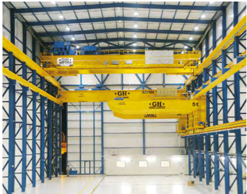
Double girder crane and cantilever crane
